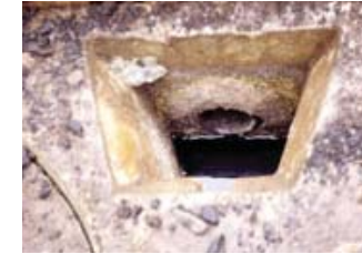
In this picture, looking down an outlet baffle, the effluent is below the pipe, indicating a bad seal.
